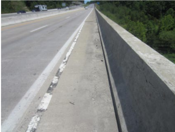
Looking east along inside face of right parapet showing debris
