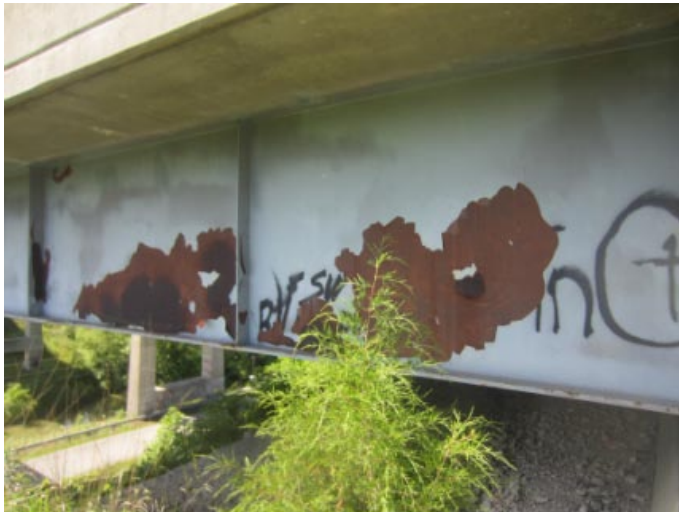
Paint flaking off outside face of right outside beam in span #3
