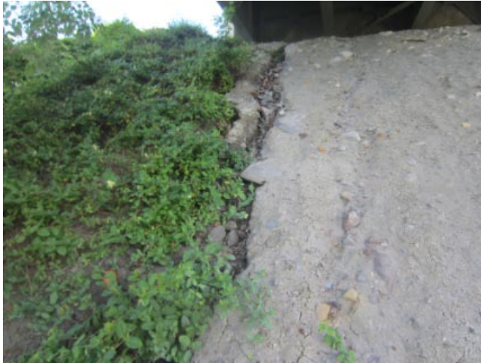
Gully washing out along left side of slope protection next to abutment #4
