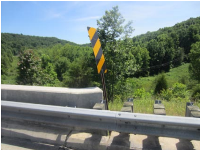
Right side obstruction marker at abutment #1
