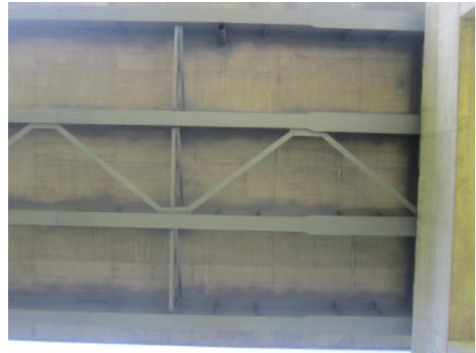
Transverse cracks in deck in span #1 next to pier
