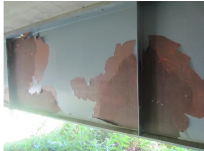
Paint flaked off inside face of right outside beam next to abutment #1
