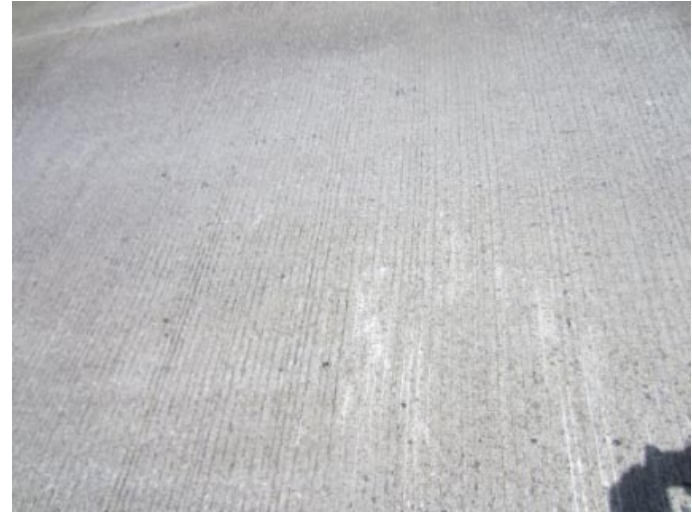
Cement seeping up through the concrete wearing surface
