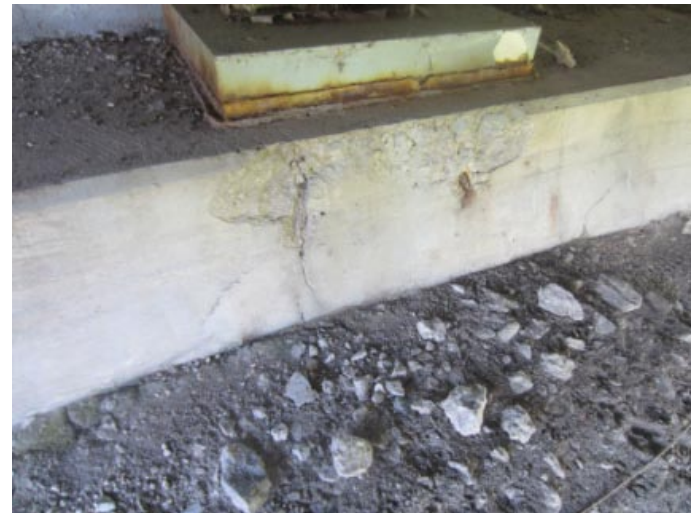
Face of abutment #4 spalling under 2nd rocker from left
