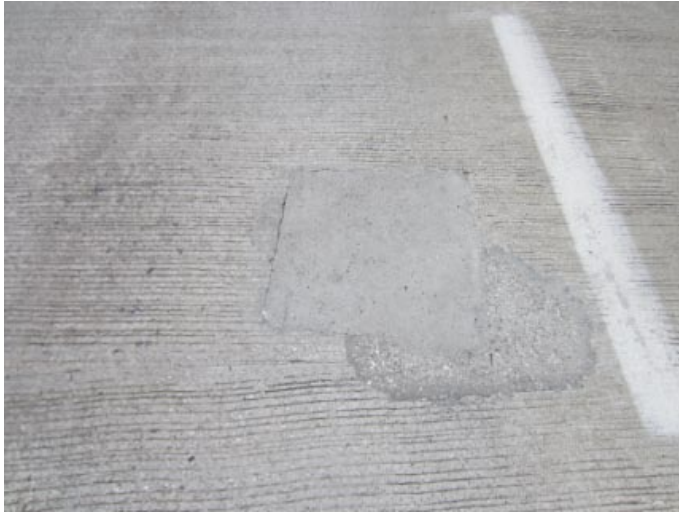
2' x 2' patched area in wearing surface in right lane
