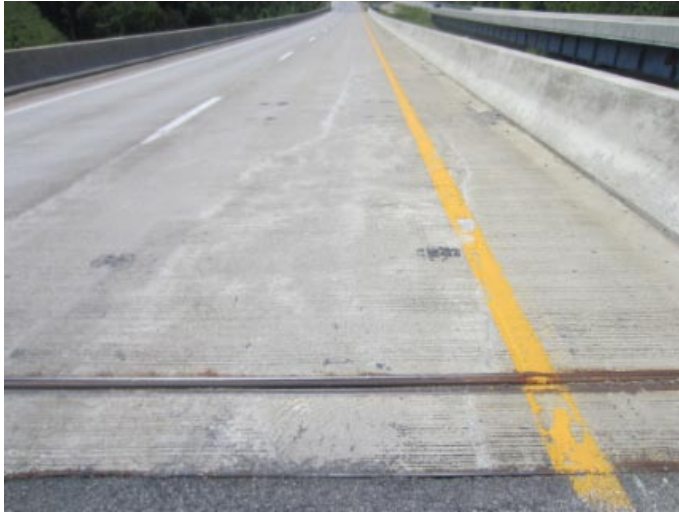
Long patched area in w.s. in left lane at east end of deck
