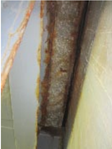
3' section of end of deck at abutment #1 has broken off lying on seat
