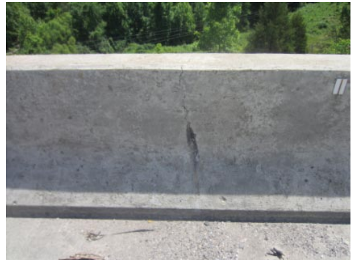
Vertical cracks in right side parapet; typical
