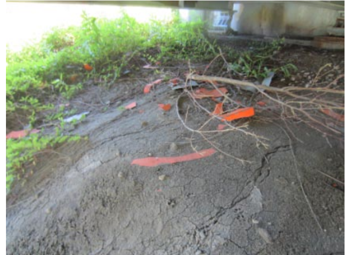
Paint flaked off beams lying on ground in front of abutment #1
