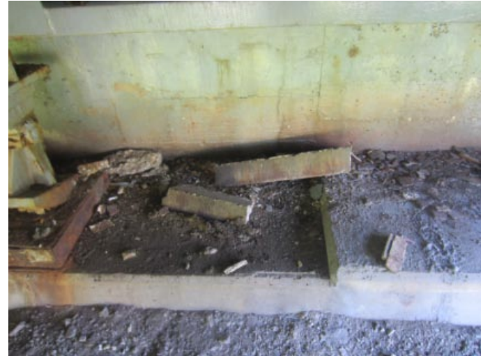
End of deck broken lying on abutment #1
