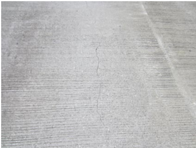
Long longitudinal cracks in right lane
