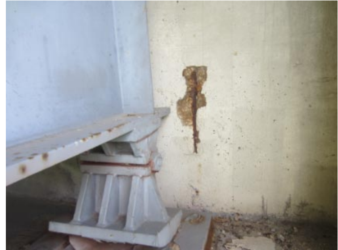
Vertical spall in #4 backwall at right end
