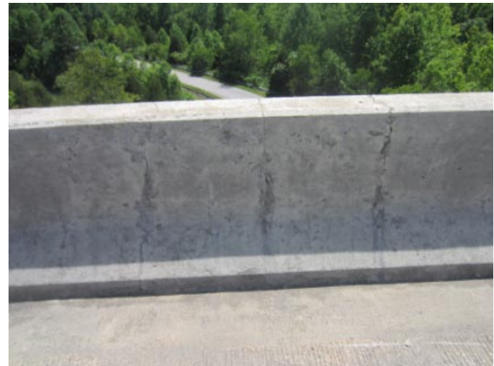
Vertical cracking in right parapet in east half of bridge
