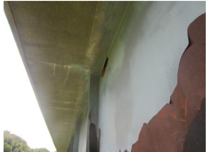
Lower outside edges of deck have transverse cracks with seepage
