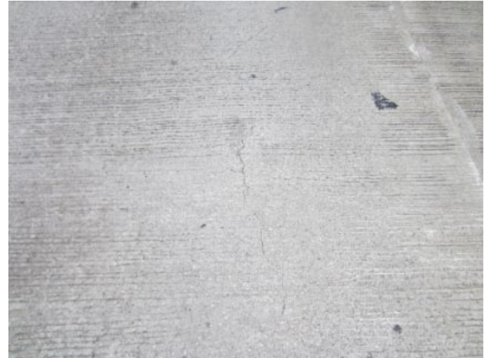
Longitudinal and random cracking in right lane
