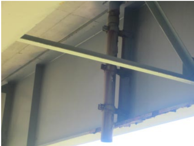
Downspout along right side rusting
