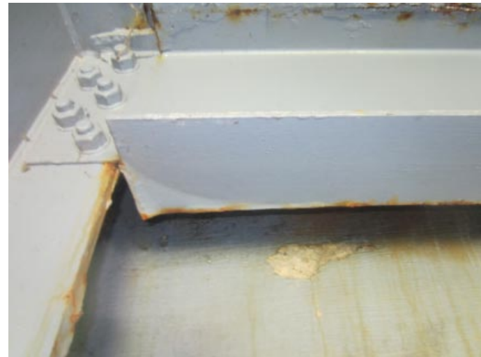
End diaphragm over abutment #1 slightly bent; very minor
