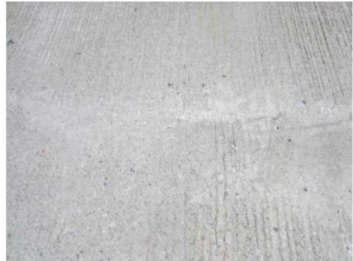
Random cracking in left lane at east end of deck
