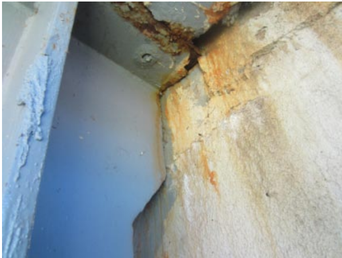
Left outside beam top flange tight against backwall at abutment #1
